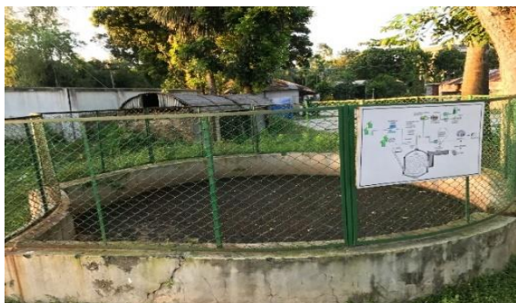
Photo: Inlet of Community Biogas Plant. Source: Najmul Huda Imran, 2017
